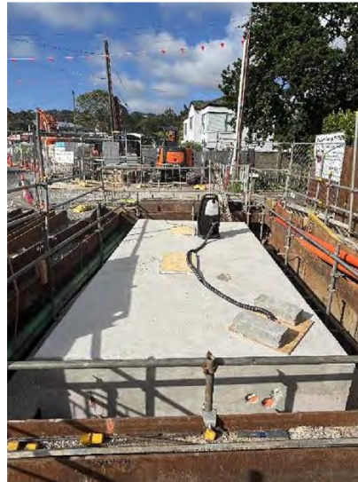
Smoke test set up for new BSP chamber
