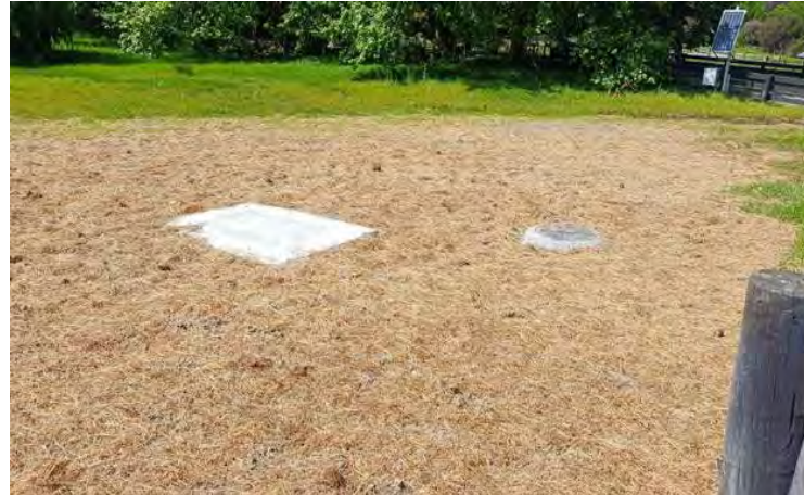
Waste collection tanks to be connected to the new Snells sewer
