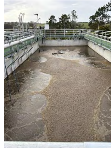
Activated Sludge Reactor in Operation October 2025
